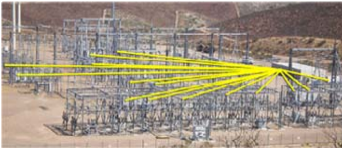
Figure 4. Telkonet Series 5 has proven performance with reliable network connectivity in various types of substations.
